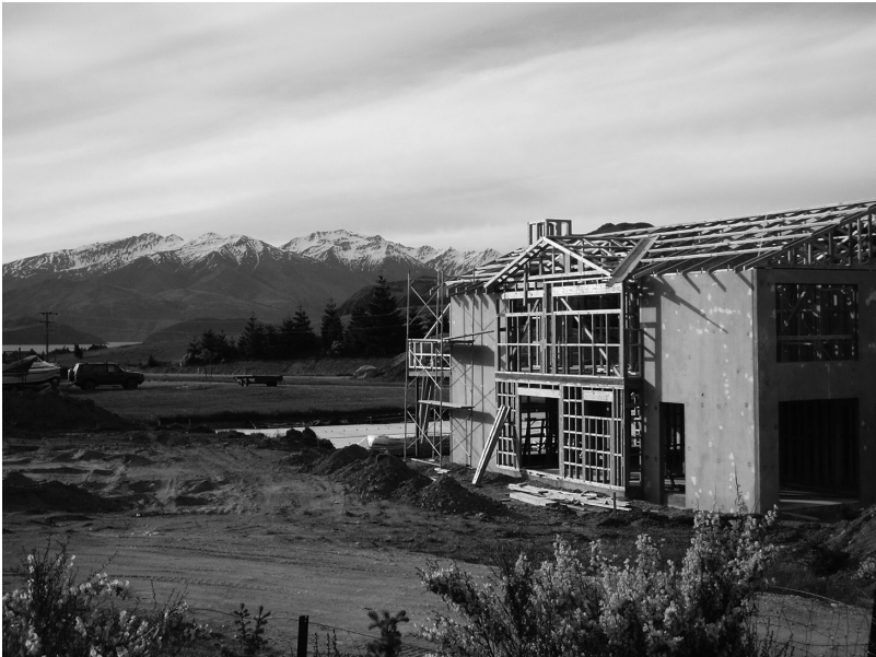
Plate 6.2 New house-building at Wanaka, New Zealand, a popular amenity migration destination (Photo: author)
